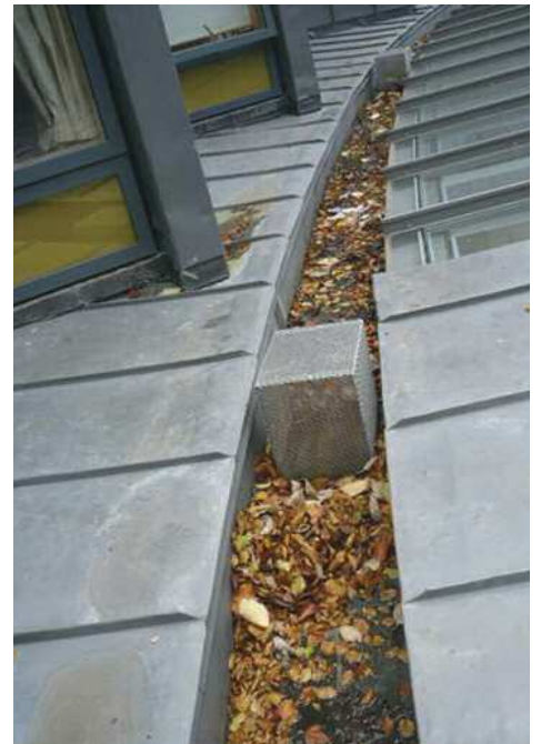
Gutters must be regularly cleaned.
