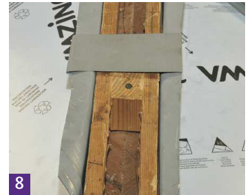
8 A zinc clip is installed prior to the hip flashing being fitted.
